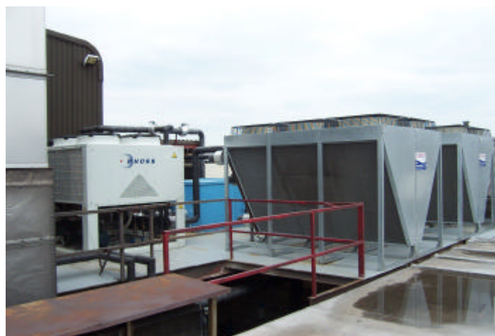
Typical air blast cooling installation
